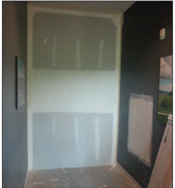
Construction is moving along at the Community Center. The new storage closet for the Art Room has been framed in. This area used to be a hallway. This will be storage for grids and sandwich boards.
